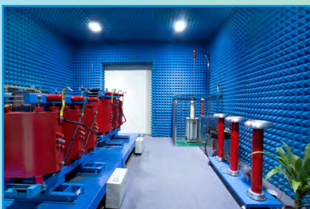
Dry transformer lab
